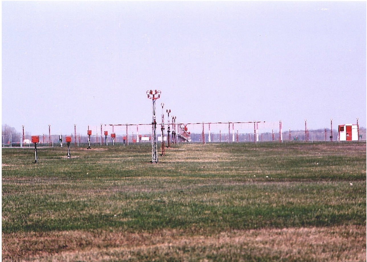
Figure 4-4. Approach lighting towers — aluminium lattice structures
