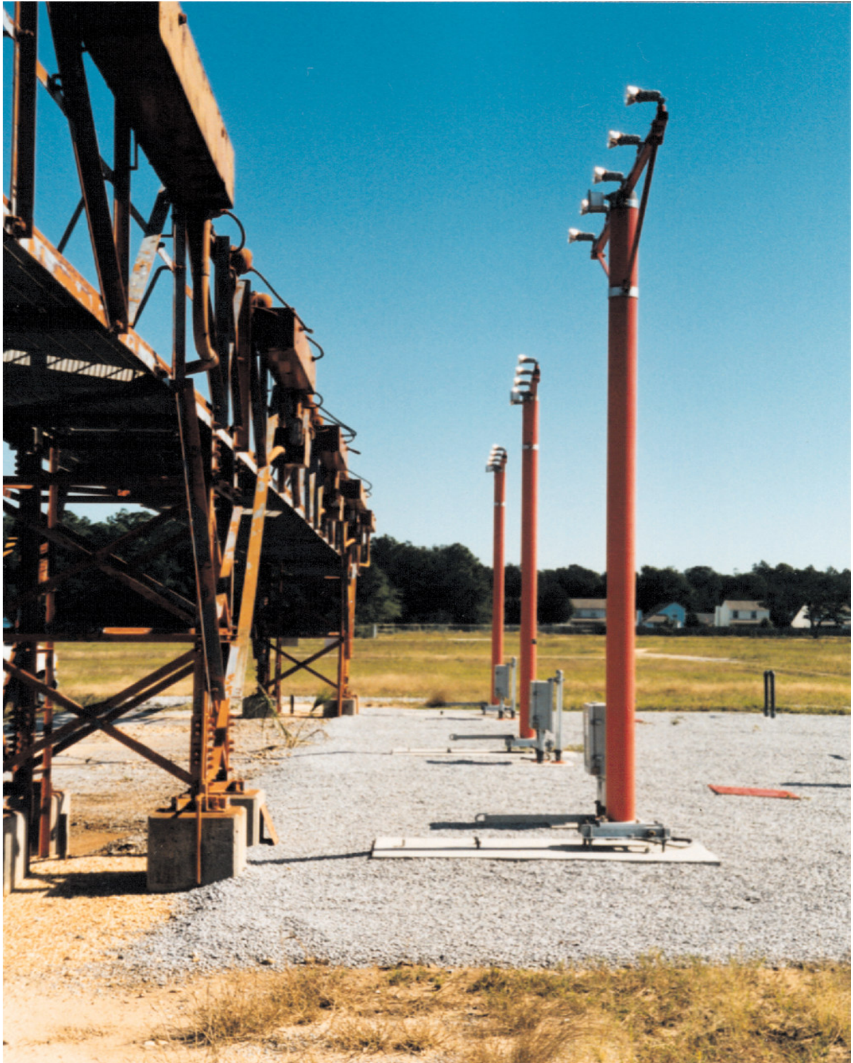
Figure 4-6. Approach lighting station of rigid design (left) being replaced by new frangible structures (right)
